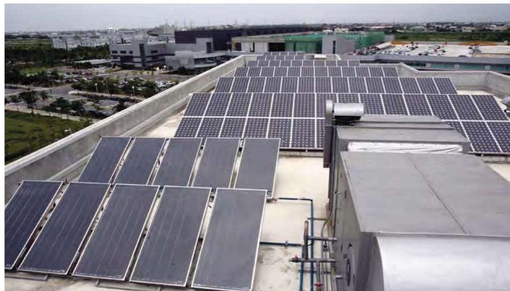
➤ Delta has installed solar panel systems and solar heating systems at facilities throughout the world.
