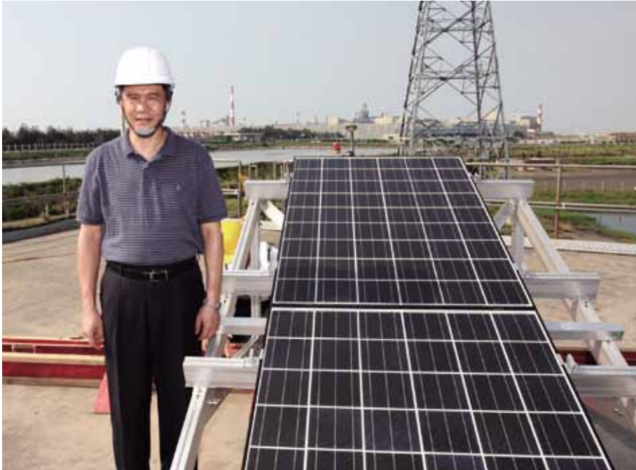
Mr. Yancey Hai with Delta's solar module on the jobsite of Taichung Fire Power Plant.
