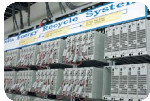
Energy recovery system installed at one of Delta's factories.
