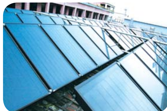
Solar water heating system installed at the employee dorm of the Dongguan factory.
