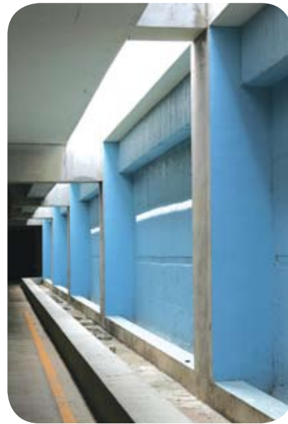
The light well at the underground parking lot at Tainan Plant is not only designed for lighting and ventilation, but is also used for rainfall recovery.
